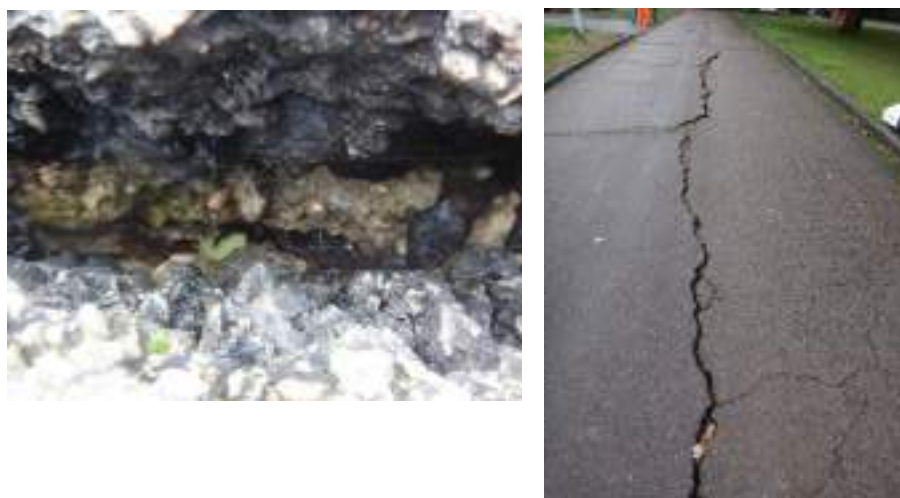
Left: view looking into crack showing asphalt & concrete layer beneath. Right: general view looking North along carriageway showing longitudinal crack along centre of road & regular transverse cracks across road surface.
