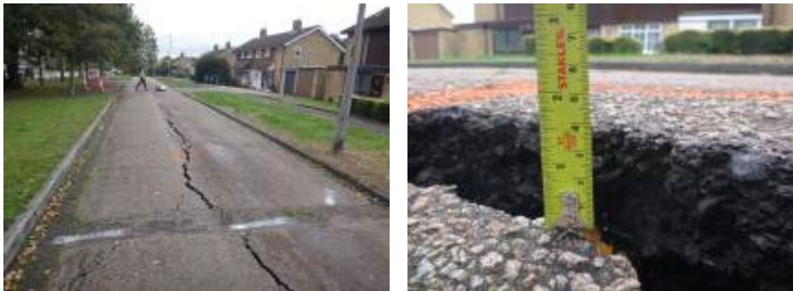
Left: General view looking South of the cracking along service road. Right: View showing the difference in surface level either side of the longitudinal crack.
