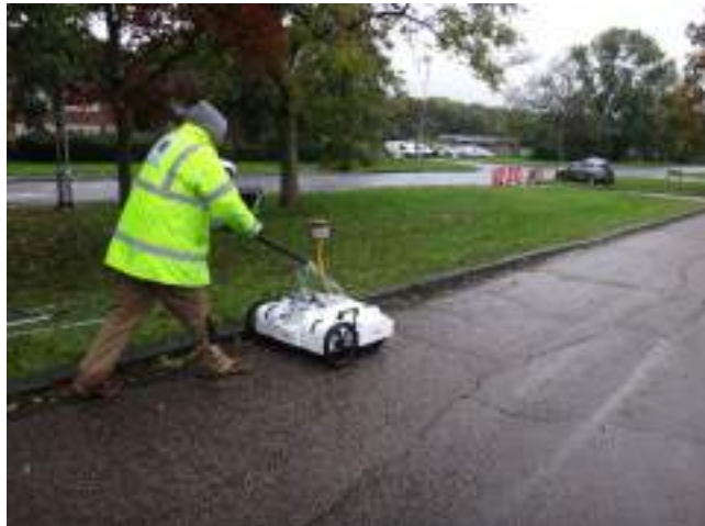
Image of the Impulse Radar Multi-channel Raptor System in use by GBG.
