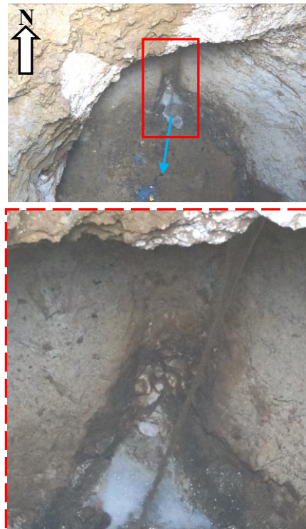
Plate 8 – Leaking Service. Flow direction shown in blue.
